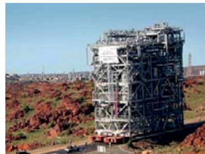
Figure 2: The world's first preassembled LNG plant by Worley Parsons, North West Shelf, Australia: an extreme example of 3rd generation modularisation.
